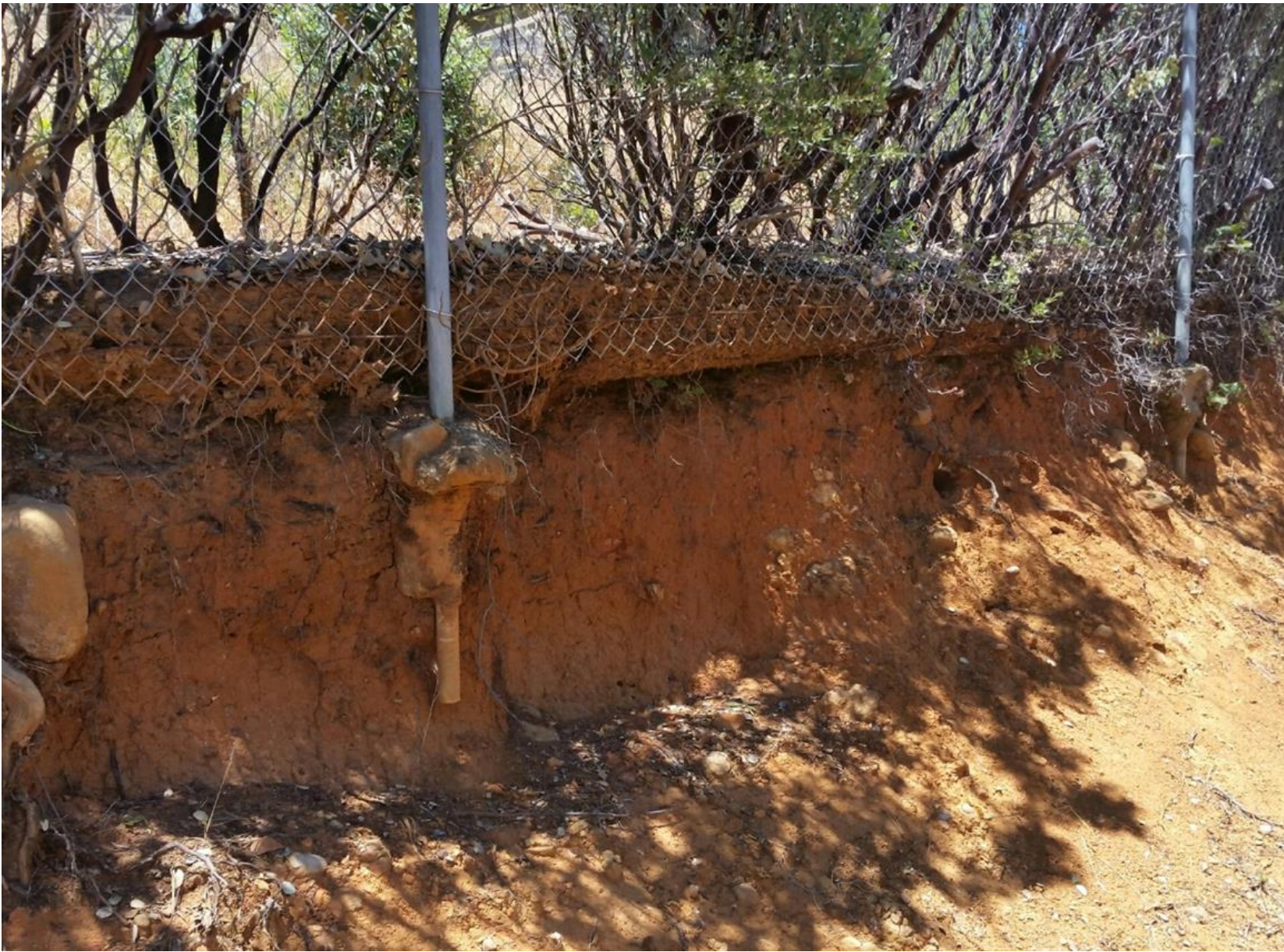
Fence at Corp Yard Erosion is 4 to 6 feet
